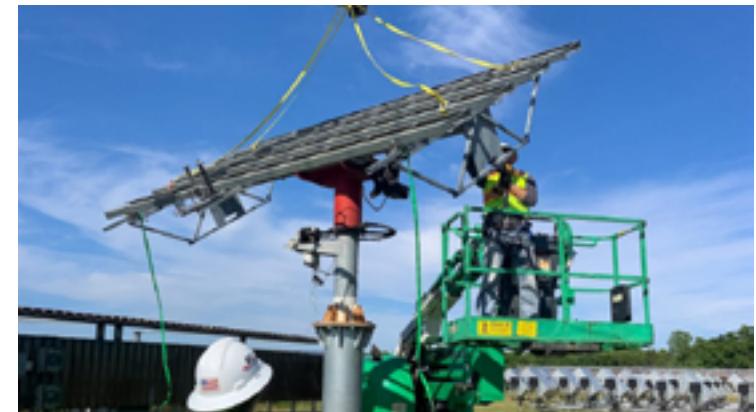
Figure 4-3. Workers decommissioning a solar facility in Catawba County, North Carolina (Credit: RCI Construction Group)
