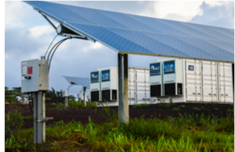
Figure 8-1. The AES Lawai Solar Project in Kauai, Hawaii, which consists of a 28 MW PV system and 100 MWh battery energy storage system and can restart the island’s electricity grid in case of an outage (Photo by Dennis Schroeder, NREL 57998)
