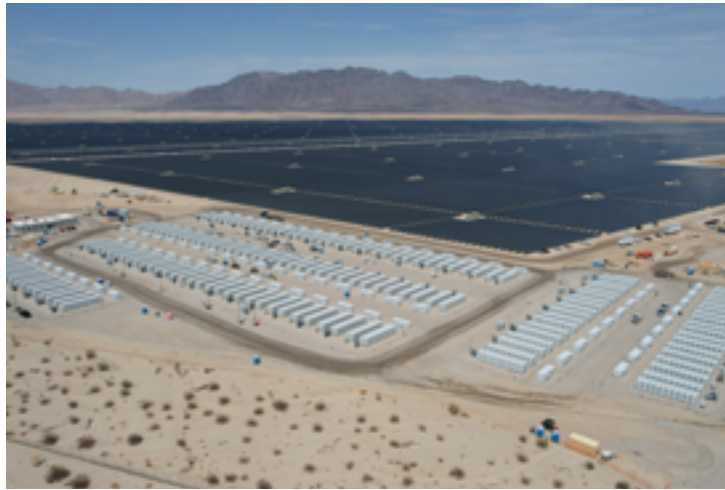
Figure 2-3. The Desert Sunlight Solar Farm, a 550 MW PV and 220 MW energy storage facility sited over more than six square miles in Riverside County, California (Credit: Bureau of Land Management)
