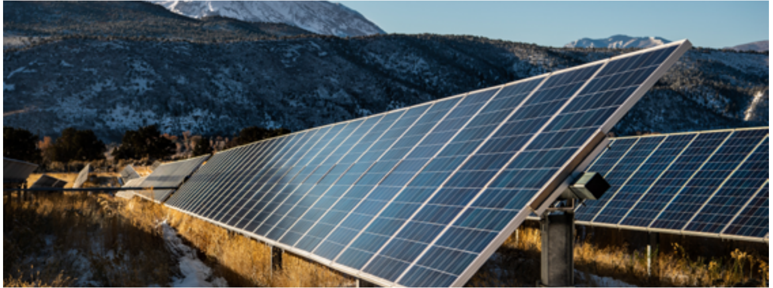
Figure 1-5. PV arrays at the Sunnyside Ranch shared solar facility, adjacent to the former Carbondale, Colorado, landfill (Photo by Dennis Schroeder, NREL 60071)
