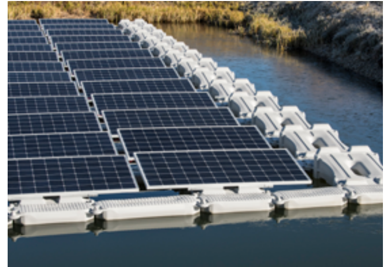
Figure 8-2. A floating PV system on a retention pond at a municipal water treatment facility in Walden, Colorado (Photo by Dennis Schroeder, NREL 53975)
