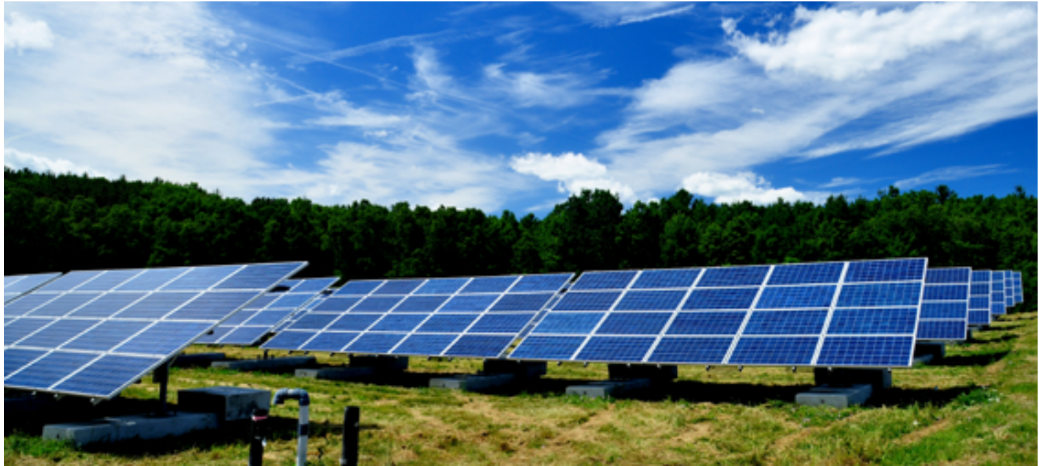
Figure 6-1. A 2.3 MW solar energy system sited on top of a closed municipal landfill in Easthampton, Massachusetts (Source: Massachusetts Department of Environmental Protection, Flickr)
