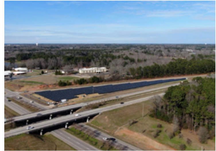
Figure 8-3. A one MW PV system at Exit 14 along Interstate 85 in West Georgia (Credit: Ray C. Anderson Foundation)
